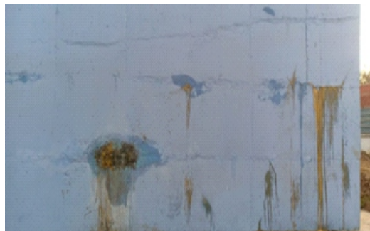
Damp and crack at Beur STP
